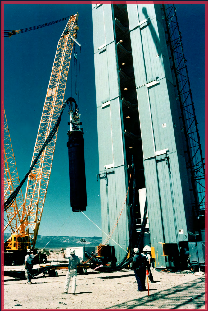
The Divider test rack during setup at the Nevada Test Site (now the Nevada National Security Site).
